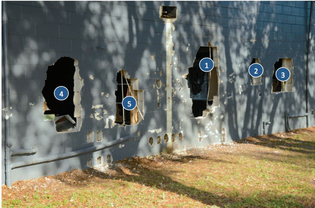
Figure 6. Breaches of Pulse nightclub exterior wall
