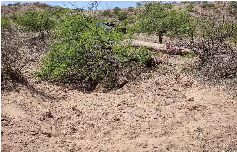
Drainage 19, Photo 3. Looking downstream, facing northwest at erosion.
