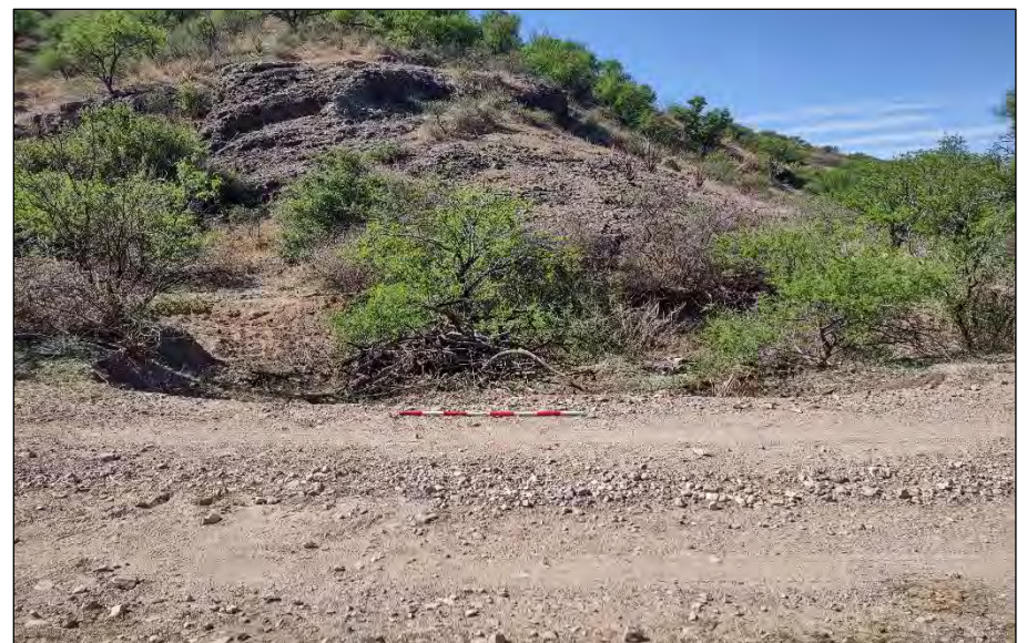
Drainage 19, Photo 4. Facing south at erosion near road (approximately 24 feet long).
