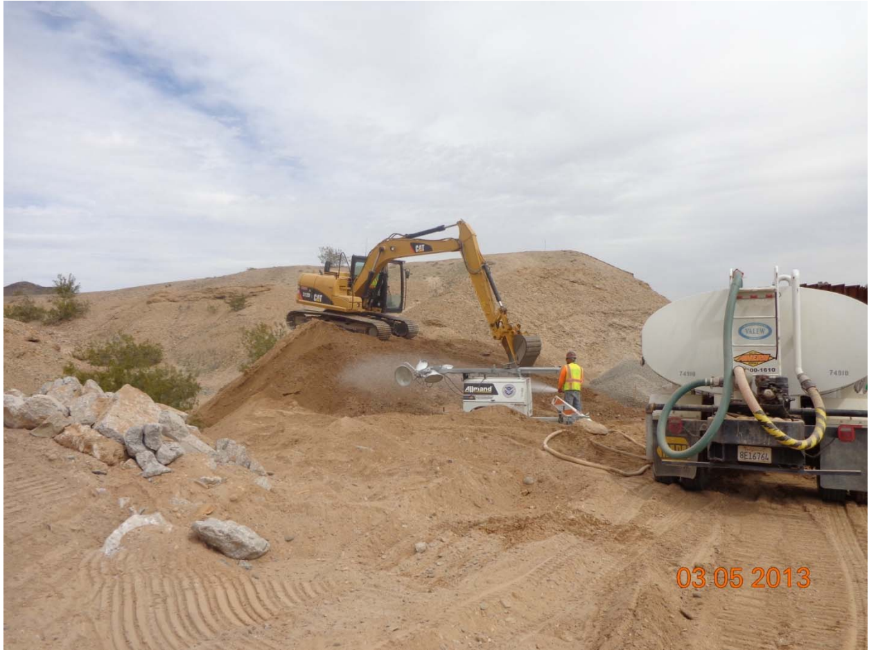
Picture 7 – CJW adding water to the engineered fill material before placement in the hole for the ramp.
