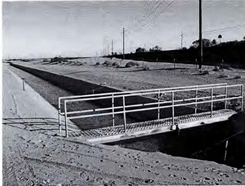
Photograph 3: Existing Footbridge over the 242 Well Field Canal looking East along the Border
