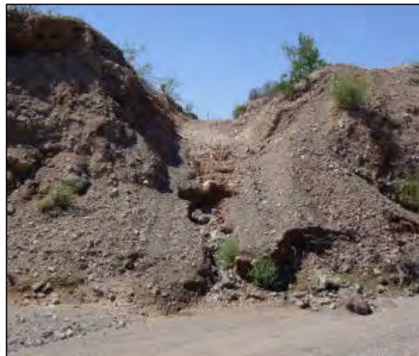
Photograph 1-16. Impassable Road Section
